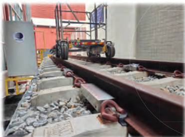
TWD sensor installed on experimental track
