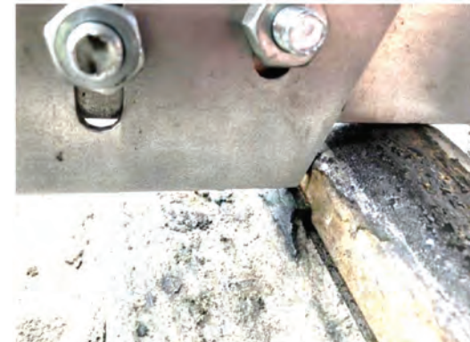
Gauge No.3, Switch No. 2, 2 in from the tongue's end, PASS or FAIL???
