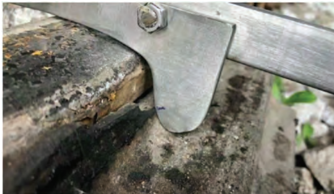
Gauge No.2, Switch No. 2, 5 in from the tongue's end, PASS or FAIL???
