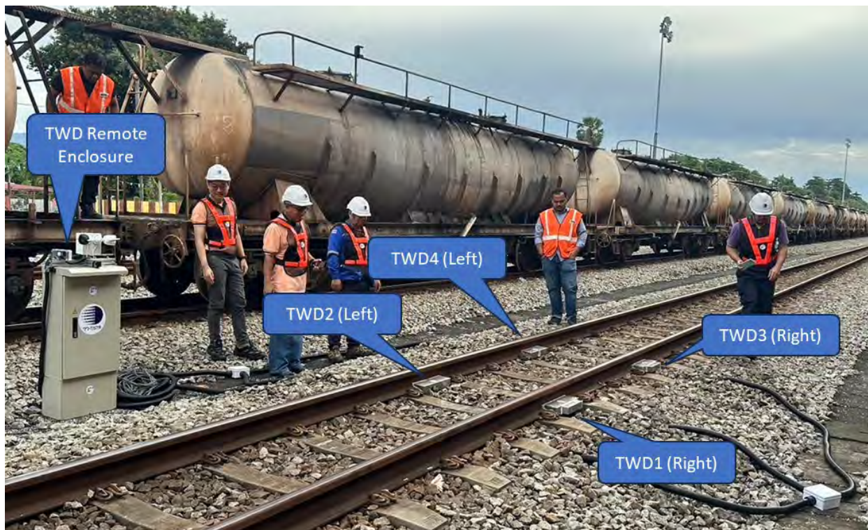
Figure 43 The TWD system is installed in the depot at Ipoh railway station.
