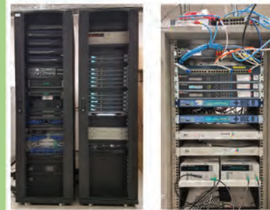
NTP server room
