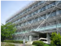
Takeuchi and Yasuda et al. applied façade and BRB to retrofit Midorigaoka building number 1, Tokyo Institute of Technology. [2]
