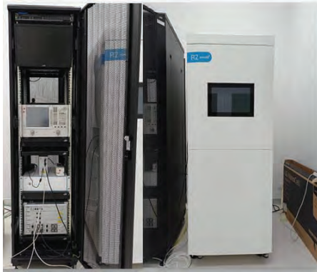
5G base station and Compact Antenna Test Range (CATR)
